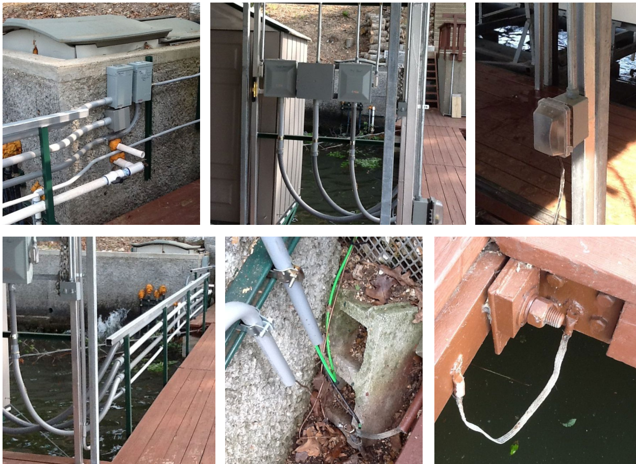
(Top Left) Disconnect at entry. (Top Middle) Mega Panel. (Top Right) GFI Covered Outlets. (Bottom Left) Conduits Anchored Flex. (Bottom Middle) Ground Rod. (Bottom Right) Bonding Jumper.
